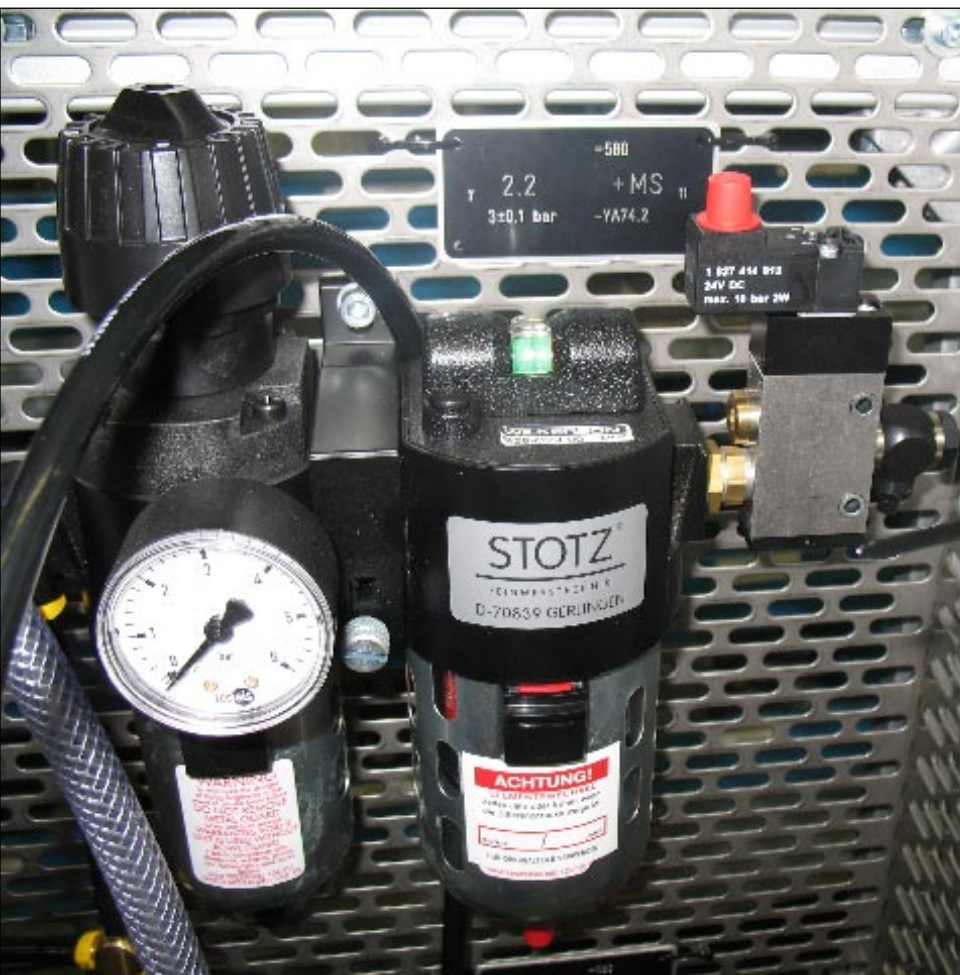
Installation illustrating a shutdown mechanism on an air compressor that reduces the air flow by 90% when the air gage is not in use, thus saving substantial energy costs for the shop.
